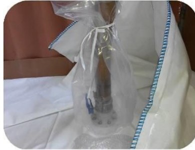
Cover the bonnet on the loading pipe, in case any spillage comes out
